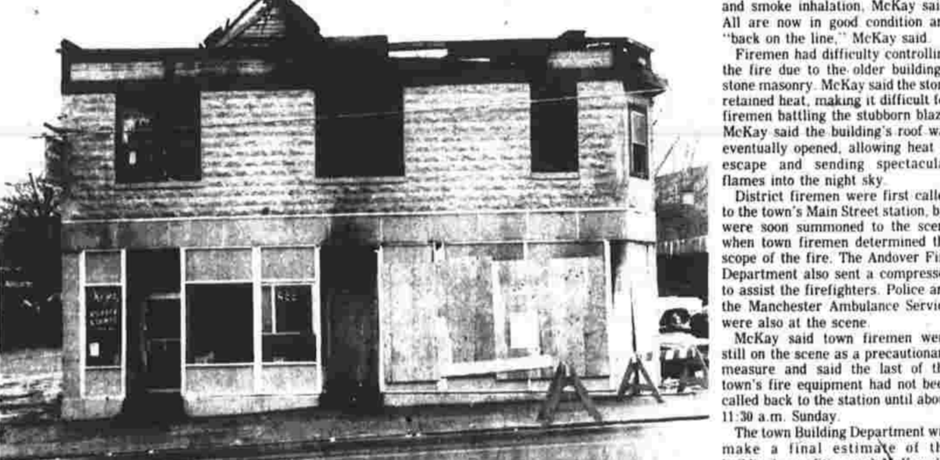
A fire early Saturday morning gutted a building at 451-459 Main St., driving six persons from their apartments and causing an undetermined amount of damage. Nine firemen sustained minor injuries, and all are back on duty. (Herald photo by Pinto)
